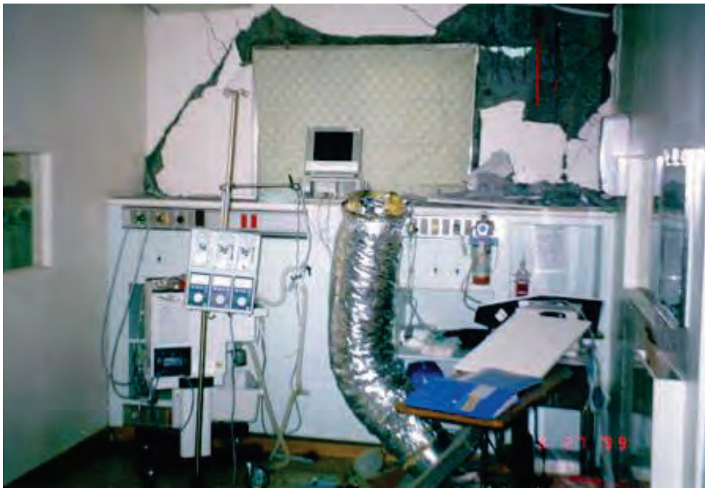
Figure C13.1-3 Collapsed duct and HVAC diffuser.
