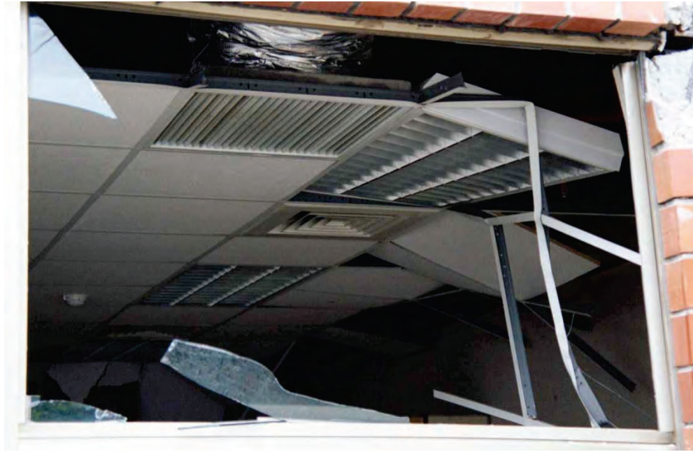
Figure C13.1-4 Damaged ceiling system.
