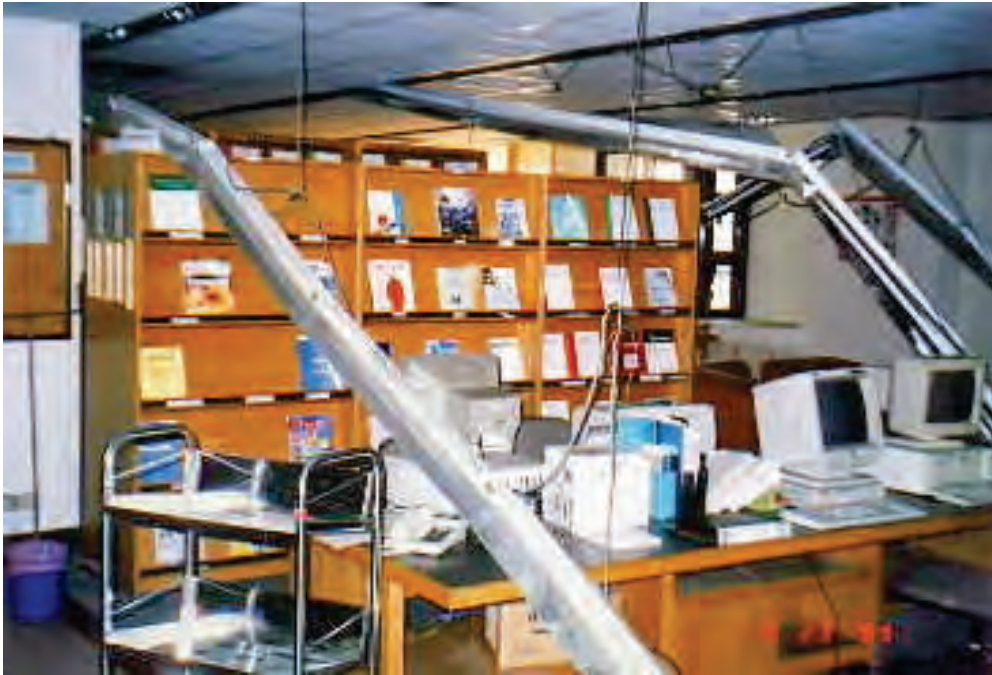
Figure C13.1-2 Collapsed light fixtures.
